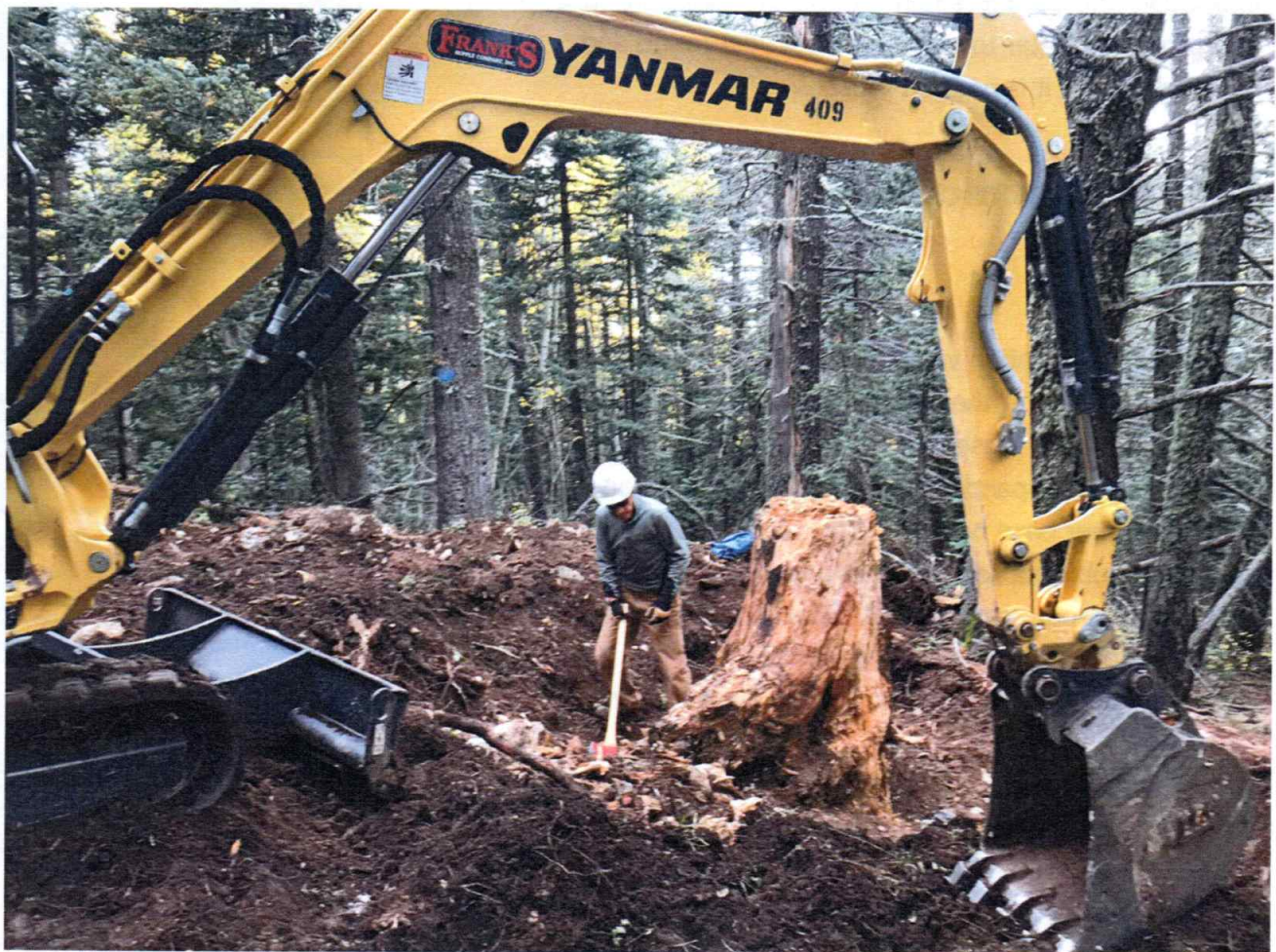
Jess Huser cutting roots of a huge stump to make it easier for the mini excavator to dig out.
