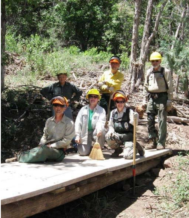
Volunteers on Repaired Cienega Canyon Trail Bridge. L to R: B. Savage, D. Carnicom, S. Lowder, B. Lowder, R. Nicholson, and S. Beard.
