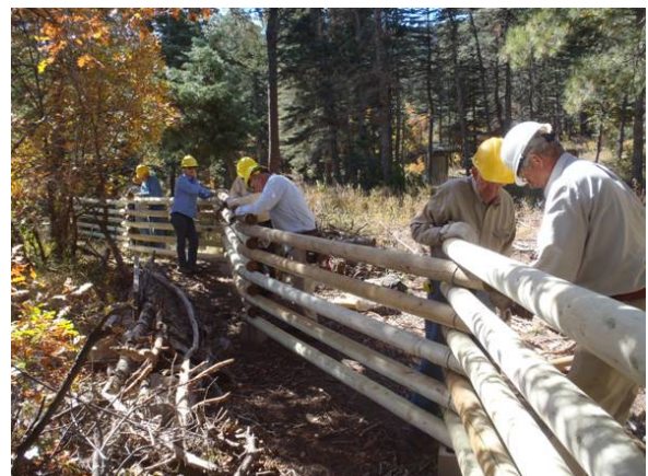
Volunteers at Tree Spring Trailhead attaching poles to the posts with wire and Larry Littlefield, L, and Jim Lunn placing the fifth pole on a fence section. Photo by Bet Gendron
