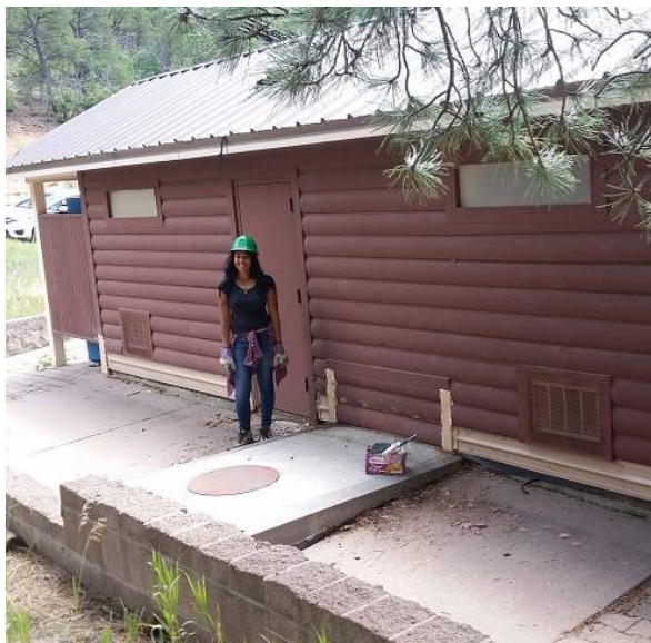
Saybell Taylor-Aboy beside Doc Long restroom where she and Gordon Eatman have replaced rotten wood with steel panels. Photo by Gordon Eatman
