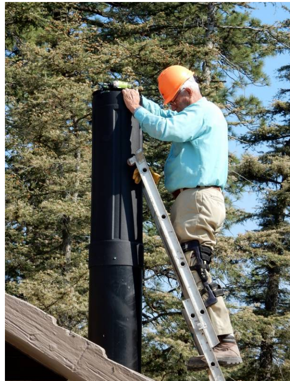
Jim Lunn installing a Poo Poo Screen on vent pipe at restroom in Balsam Glade Picnic Area. Photo by Dan Benton
