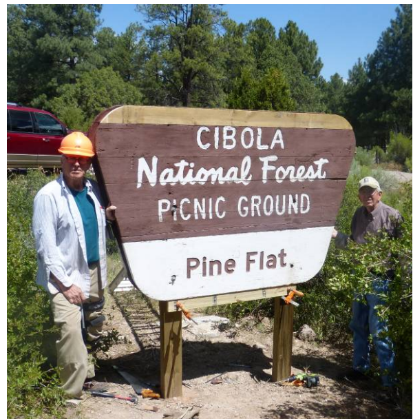
Installation of repaired sign at Pine Flat PA. L to R: Jim Lunn and Larry Littlefield. Photo by Sam Beard
