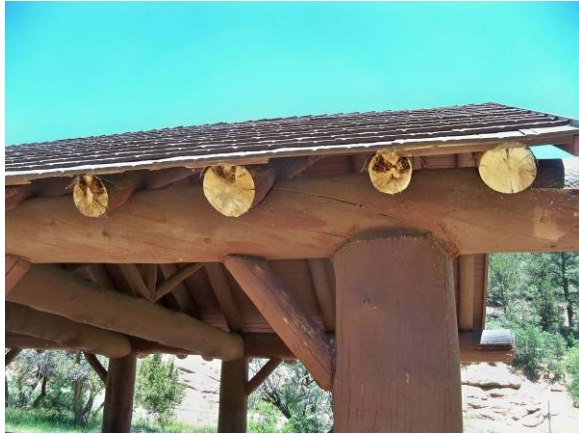
Ends of cut vigas on picnic shelter in Doc Long Picnic Area. Brown color indicates rotten wood. Photo by Sam Beard
