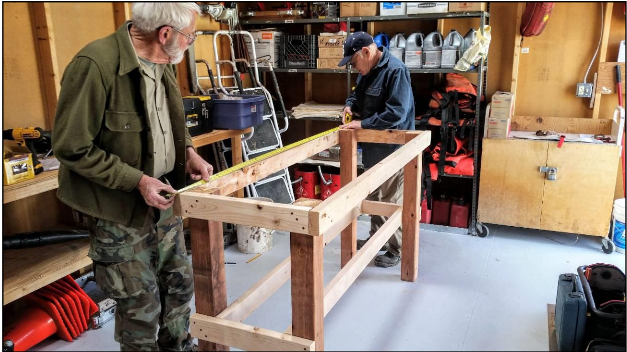
Sam Beard and John Torres building the heavy-duty work bench in the FOSM Guard Station. Photo by Betsy Galloway
