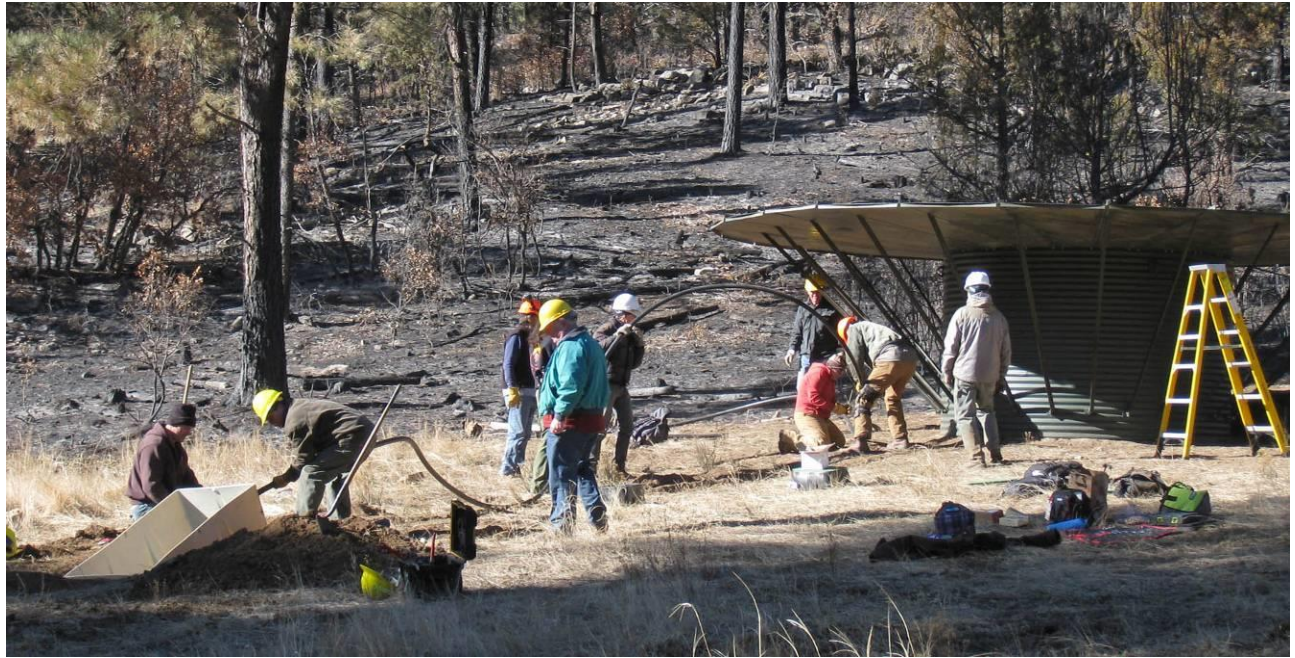
The FOSM crew installing the water pipe from the tank to the drinker at the David Canyon West Wildlife Drinker. They have already completed the installation of the wings on the rain collector on the right. Note that the forest has been burned as part of a thinning project. Photo by Carl Smith
