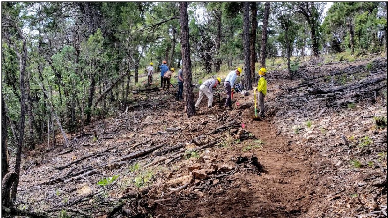
The crew snakes up a ridge building a new section of trail. Photo by Betsy Galloway
