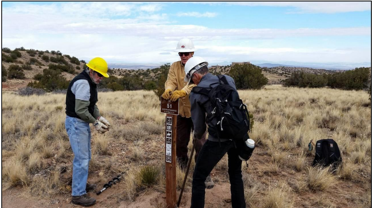
Byron Garner and Sim Cook pack rock backfill around the post while Casey Cook holds the sign in position. Photo by Betsy Galloway
