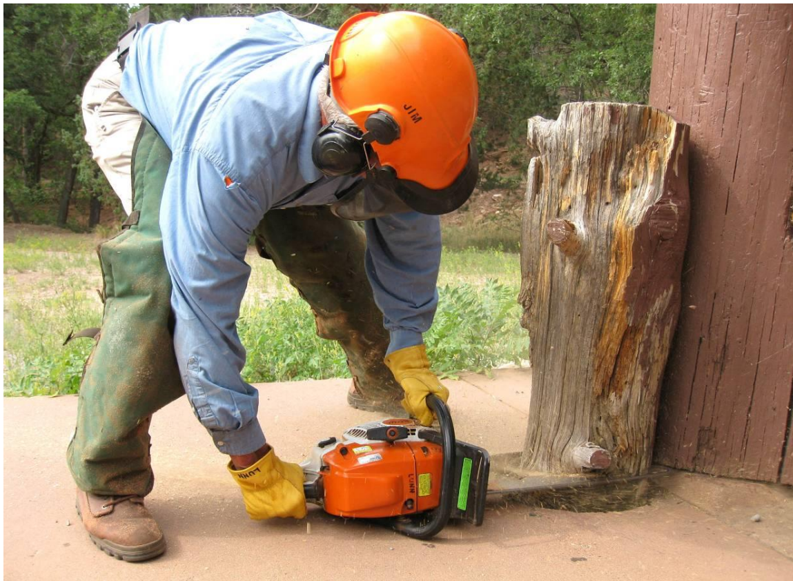
Jim Lunn is using his chain saw to low cut a decayed decorative post on Modern Shelter A in Doc Long Picnic Area. The decayed wood below the cut was eventually removed so that the hole could be filled with concrete to eliminate the tripping/falling hazard. Photo by Carl Smith
