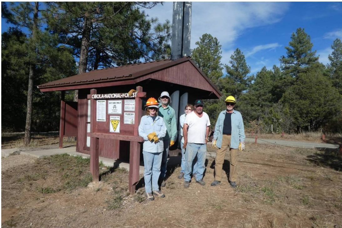
L to R: Betsy and Bob Galloway, Ellie and Russell Parker, and Dan Benton after they completed the new steel roof on the Pine Flat PA north restroom. Photo by Sam Beard
