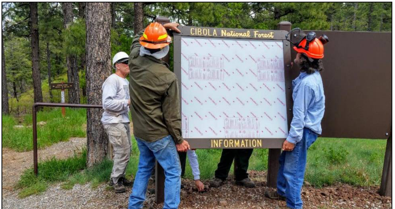
Volunteers install the kiosk information panels at the Cienega Horse Bypass Parking Lot. Photo by Betsy Galloway.
