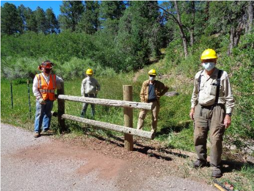
Top – Two posts replaced in Cienega PA. L to R: Dan Benton, Don Carnicom and Dennis Crowther. Bottom – One post replaced in Sulphur PA. L to R: Dennis Crowther, Jerry Carroll, Dan Benton, and Sam Beard. (The SRD map indicates that this drainage is Sulphur Spring.)
