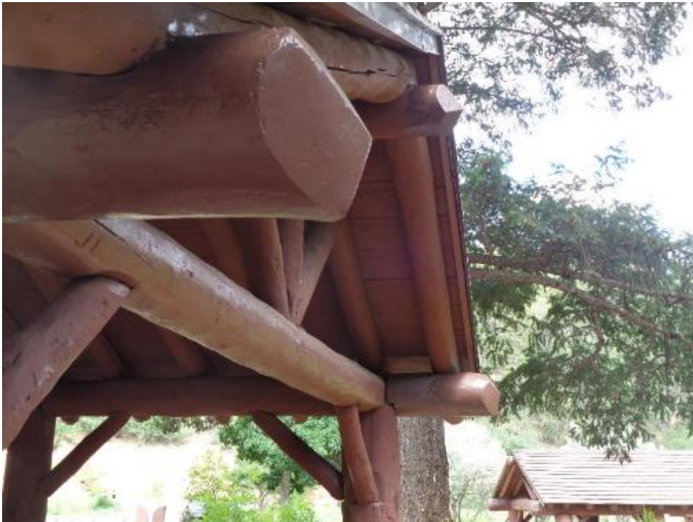
South end of the CCC shelter in Doc Long Picnic Area with three restored beams -- two large horizontal beams and the ridge pole.
