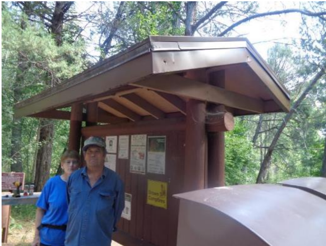
Ellie and Russ Parker are standing at the large kiosk across Cienega Picnic Area Road from the second restroom. The decayed wooden fascia in the top photograph has been covered with a custom-made brown sheet steel feature that will prevent further decay and be attractive.
