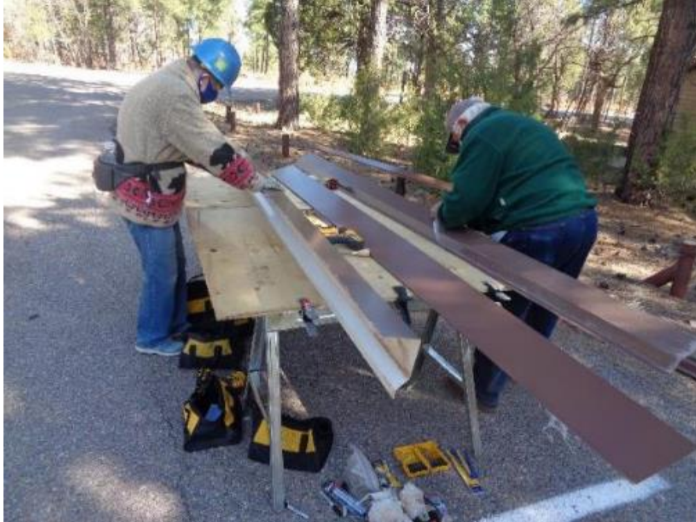
Ellie Parker and Lou Romero peeling the protective plastic film from gable trim for a metal roof on a restroom in Oak Flat Group Picnic Area.
