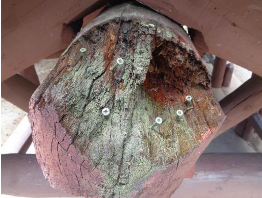
North end of ridge pole showing damage due to exposure to weather for 85 years. Screws provide anchors for epoxy putty that will be placed on the beam to restore its original shape with three flat facets.
