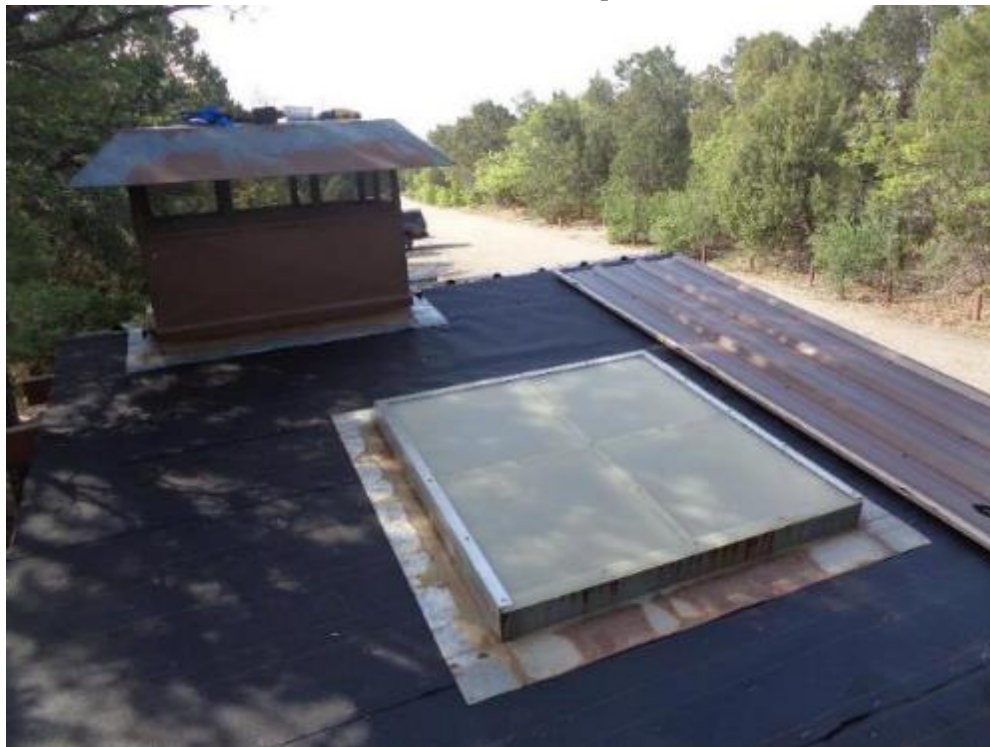
A restroom roof in Oak Flat Picnic Area showing the ventilation structure, black felt underlayment, skylight, and one brown steel roofing panel.
