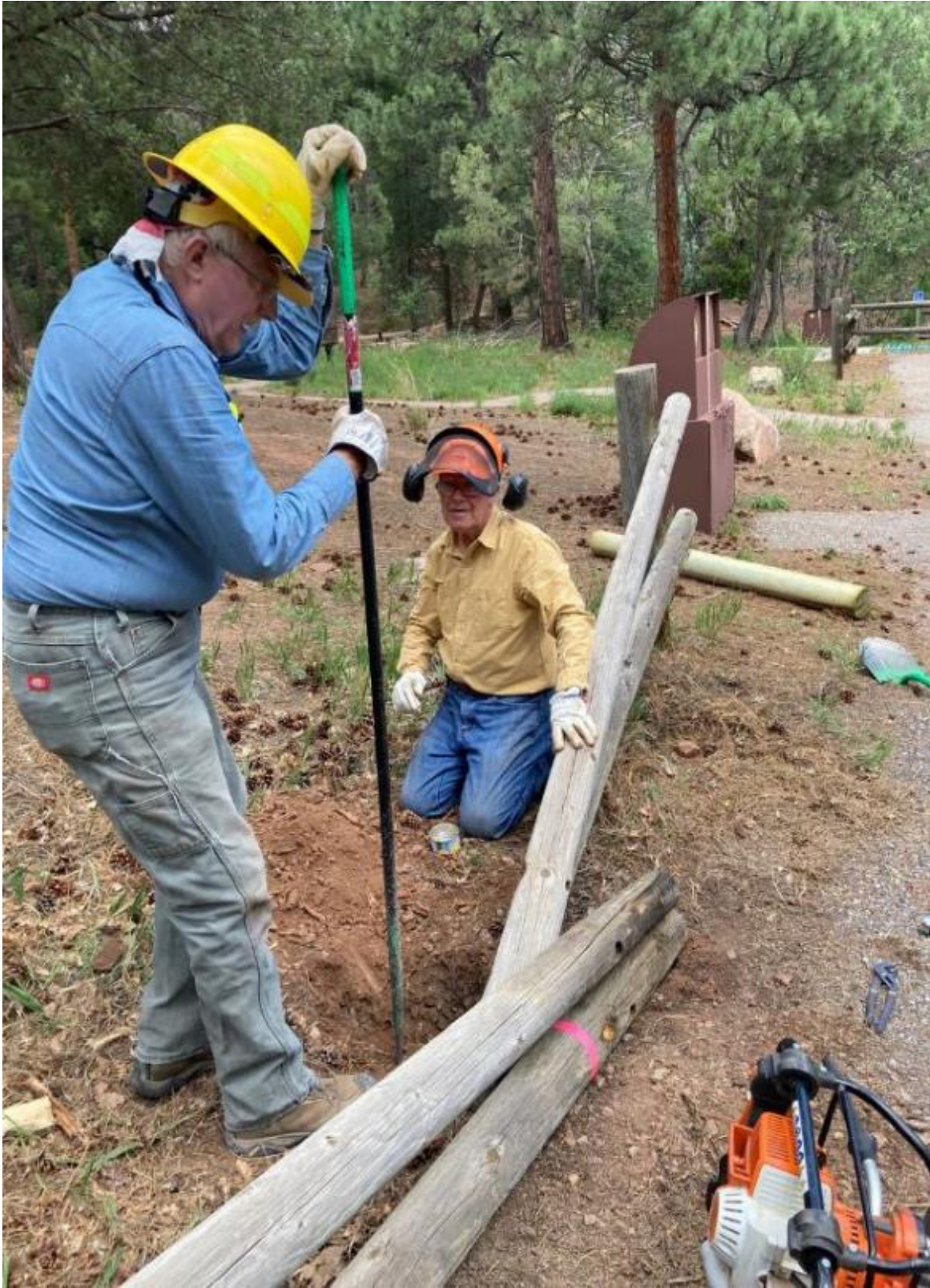
Eric Russell is using a steel bar to remove the buried part of a fence post that broke just below the surface in Cienega Picnic Area. Jerry Pekarek will remove dirt and wood fragments from the hole.
