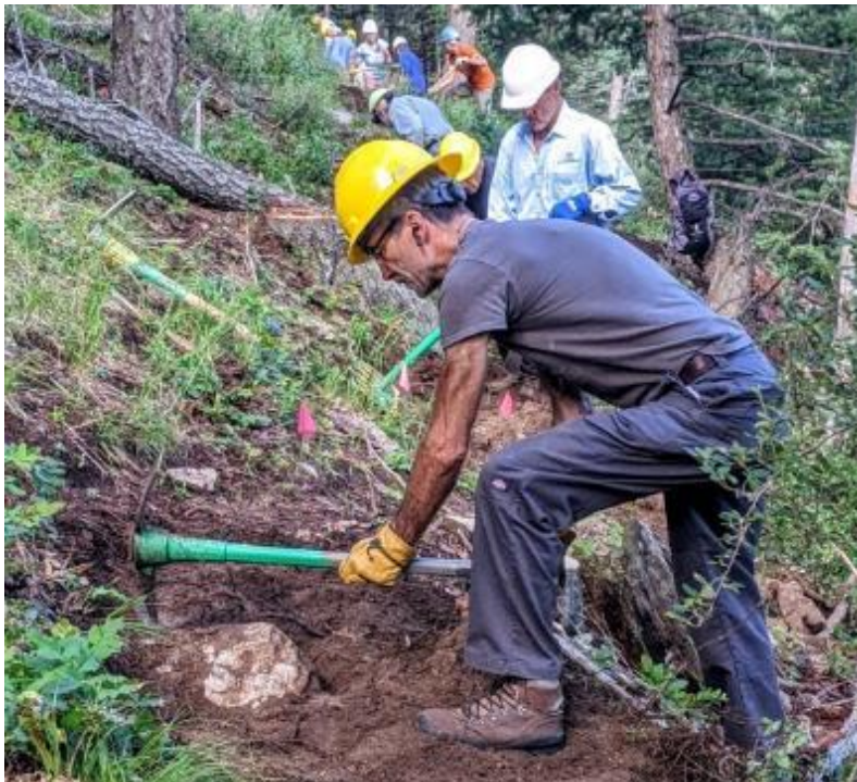
The Trail Construction Crew lines up along the Challenge Trail Extension with Roland Stumpf and Tony Pachelli in the foreground.
