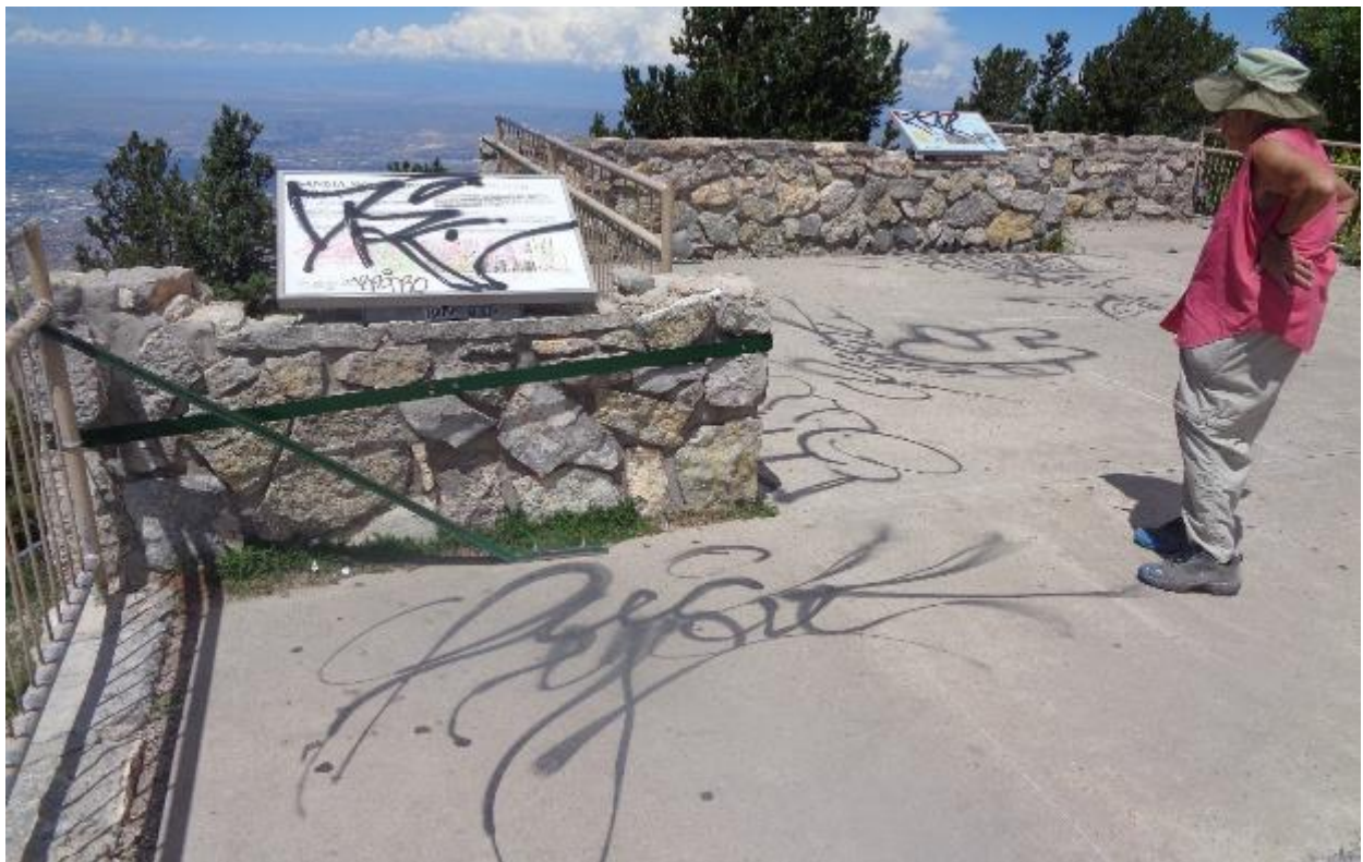
FOSM volunteers installed the supports for the railing on the left at the Crest Observation Deck so that visitors would not fall off the deck if the loose railing failed. They anchored the angle support to the concrete deck. The horizontal steel support was anchored to the stone wall and a railing post on the other side of the wall. The USFS removed the graffiti later.
