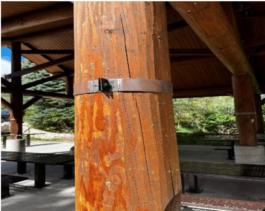
Large wooden column in Capulin Picnic Area Shelter secured with two steel bands and two bolts.
