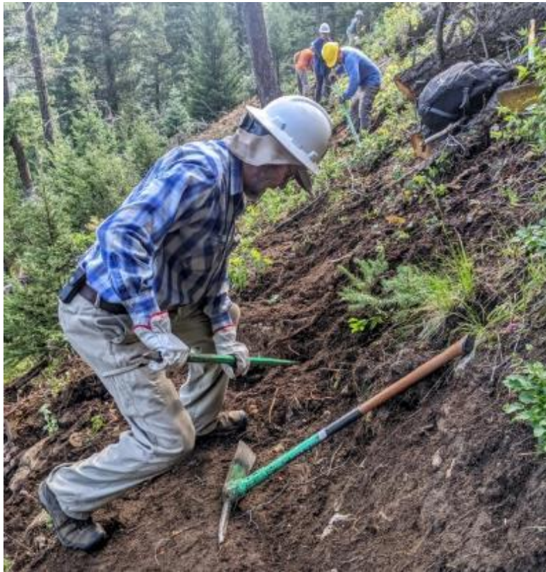
Bruce Hansche works to remove a rock on a steep section of the Challenge Trail Extension south of Tree Spring Trail, with Ralph Kopp and other trail construction crew members in the background.
