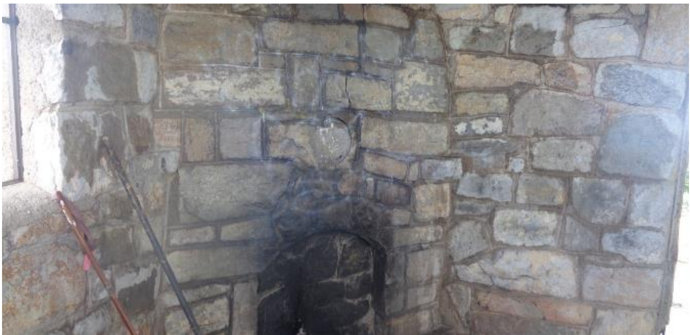
After the chemical and paint residue have been washed off with water, most of the graffiti has been removed.
