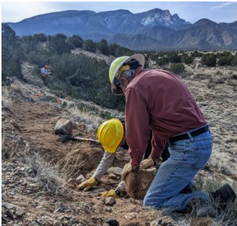
Byron Garner and Sim Cook do some rock work while building a new trail in the Placitas Trail System.
