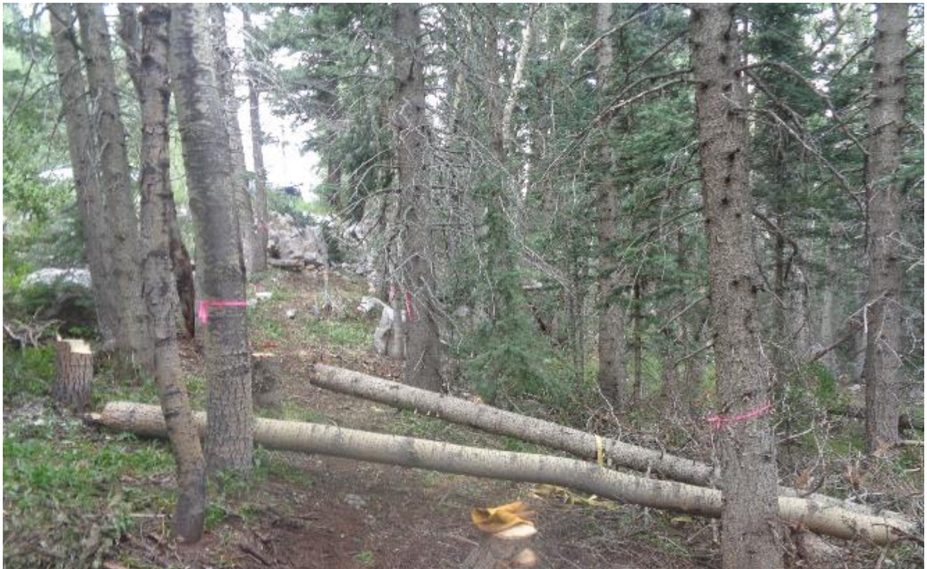
The north end of the Klaus Trail reroute where one cork bark fir was leaning on a neighboring dead fir, and the sawyers decided to fell both trees together.
