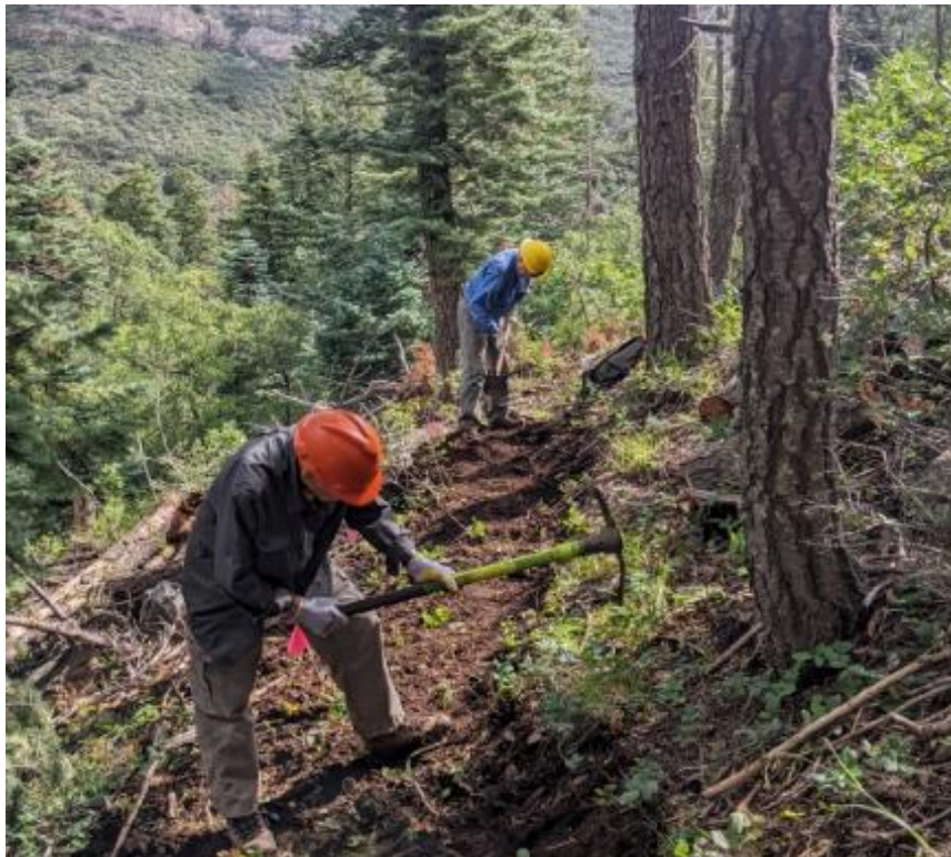
Don Carnicom and Eric Russell build new trail on the Challenge Trail Extension south of Tree Spring Trail.
