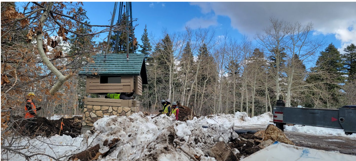
Forest Service Photo: Installation of a new vault toilet at Sandia Ranger Districts 9 Mile Recreation site.
