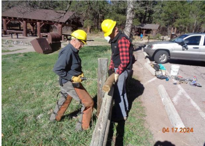
Dan Benton and Sim Cook replacing a broken fence pole in Doc Long Picnic Area
